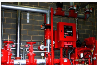
Fire Hydrant System
