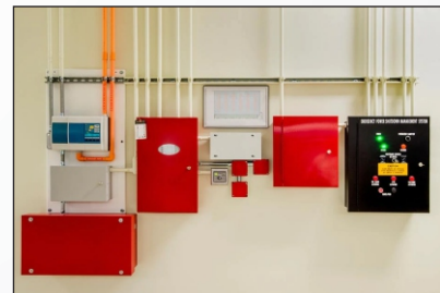
Fire Detection System
