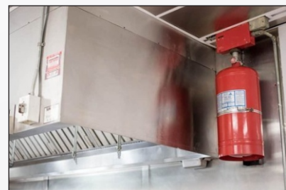
Kitchen Fire Suppression System
