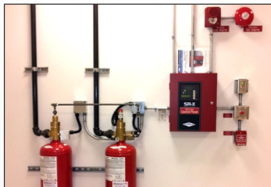
Clean Agent Fire Suppression System
